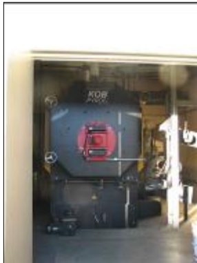
Picture 1: KOB – European high efficiency wood combustion boiler in Edmonton
